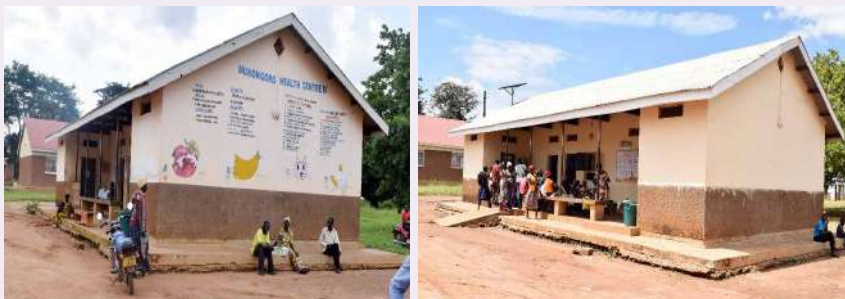
Mukongoro Health Center III in Kumi District before (on the left) the construction of the ramp and after (on the right) to ease access by persons with disabilities and the elderly
